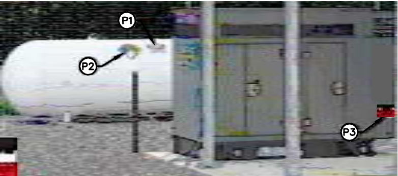
FIGURE 7 – PROPANE TANK & GENERATOR SIGNAGE
