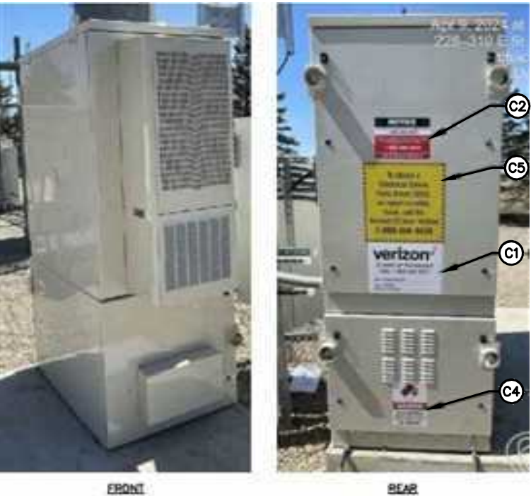
FIGURE 1 – EQUIPMENT CABINET SIGNAGE
