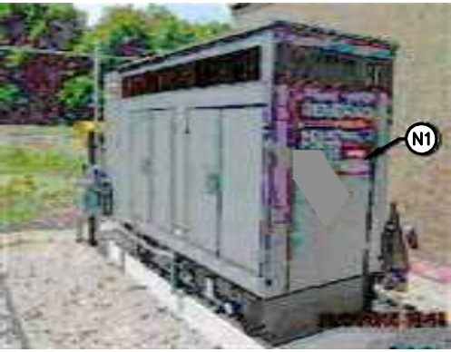
FIGURE 8 – NATURAL GAS GENERATOR SIGNAGE
